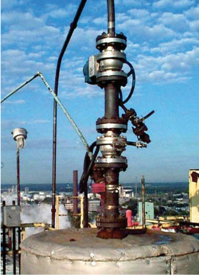
Located at the top of a major refinery, these MOGAS valves were chosen for their performance and low maintenance. Due to their location, reliability was a critical part of the installation decision.
