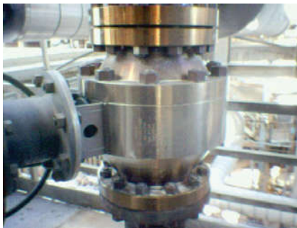
This CA-DRI 8-inch ASME 300 class valve has been handling catalyst at 1425° F / 774° C for numerous years. It is the major isolation valve between the third stage and fourth stage cyclone separator.
