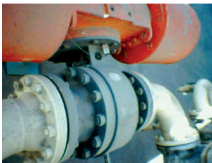
This CA-1AS 6-inch ASME 300 class feed isolation valve is a critical part of the emergency shutdown system.
