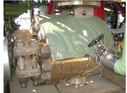
Located in a frigid Scandinavian environment, this large bore ASME 4500 class metal seated ball valve is installed on the outlets of the hydrogen heater.
