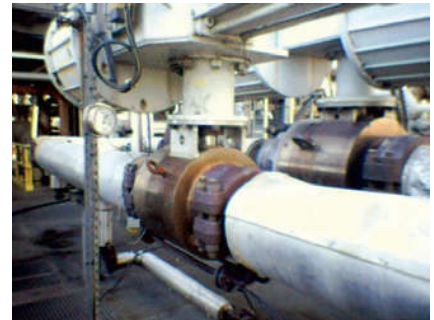
These 12-inch and 16-inch ASME 2500 class floating ball valves are installed at the letdown station of a European refinery responsible for producing 115,000 bpd.
